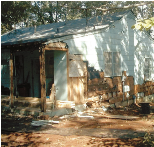
Figure 17. The siding was removed from the porch and an exterior wall of this house to show the extent of termite damage.
