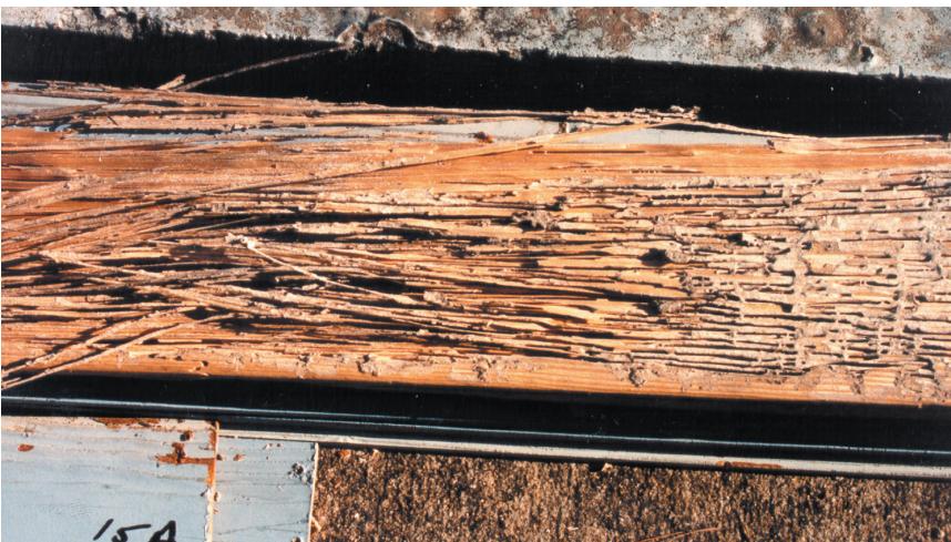
Figure 1. Subterranean termites excavate galleries in wood as they consume it, sometimes leaving nothing more than a thin wooden exterior.
