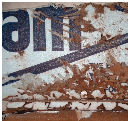
Figure 14. An example of foam-board insulation riddled with termite galleries.
